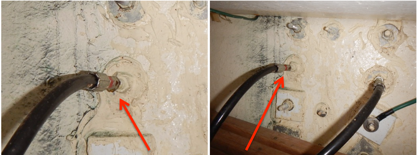
Hydraulic drip at Freedom Lift hydraulic line fitting
