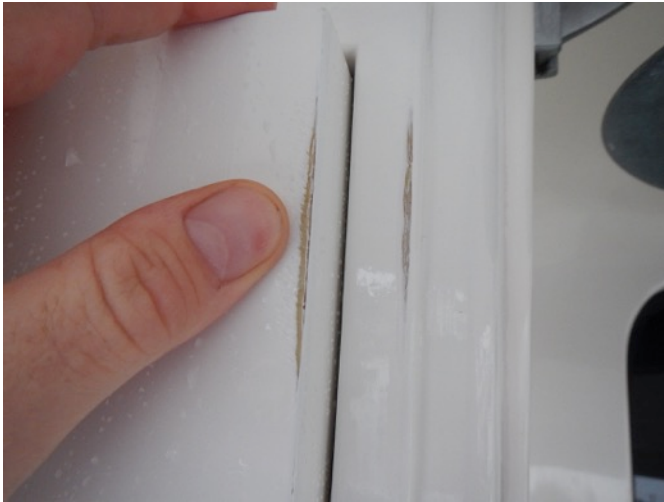
Gelcoat scratching at salon doorframe
