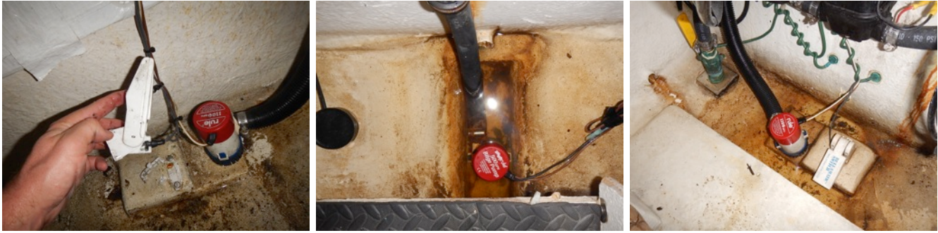
Inoperable bilge pump systems
