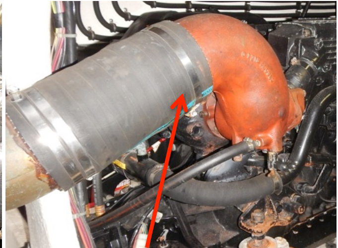
Single hose clamp fastener at main engine exhaust hose
