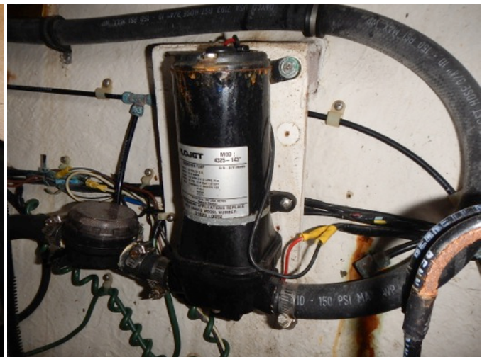
Raw water washdown pump is inoperable
