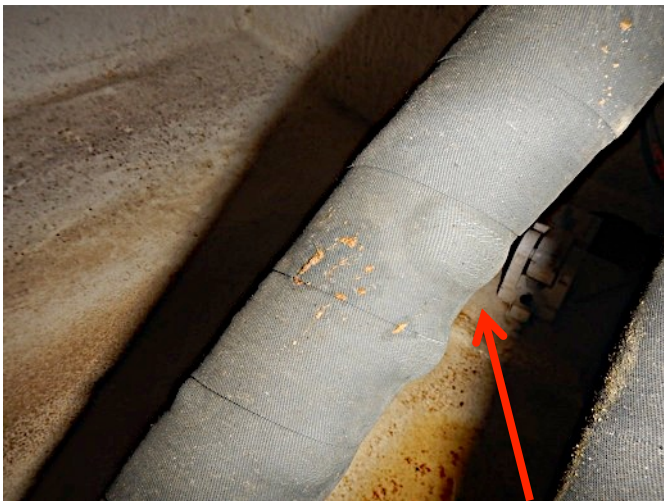
Sanitation system hoses are bulging
