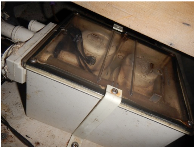
Shower sump pump is inoperable
