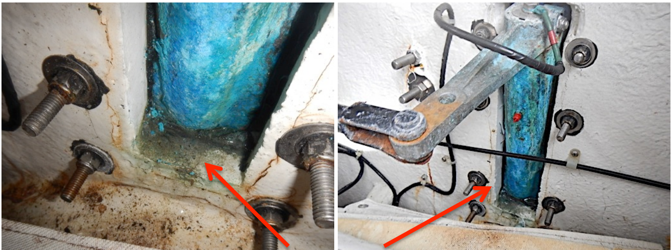
Water leak at rudder assembly to transom seal
